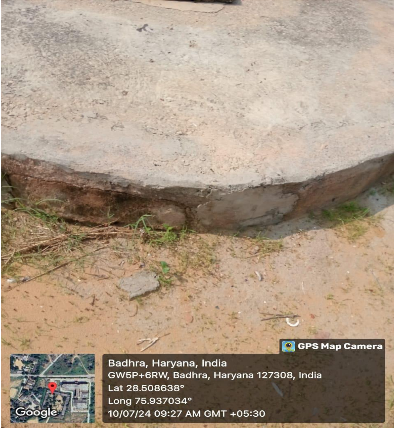
Rain water harvesting installed in the campus to raise the ground water
